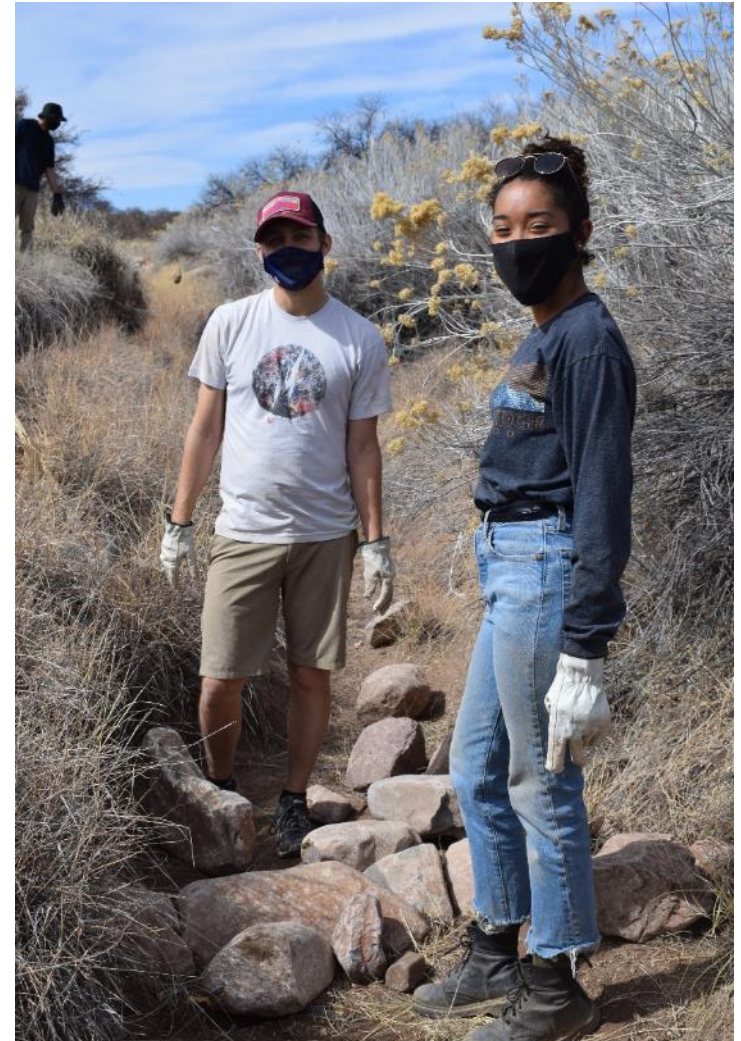
WMG volunteers build one rock dams to slow and sink flows in Empire Gulch – a tributary to Ciénega Creek. Spring 2021.
